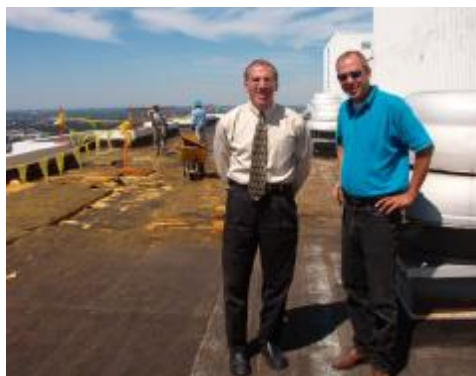
Malibu East Association Manager Vito Senese and Mark Rudolph of Winward Roofing & Construction inspect the roof replacement project.
